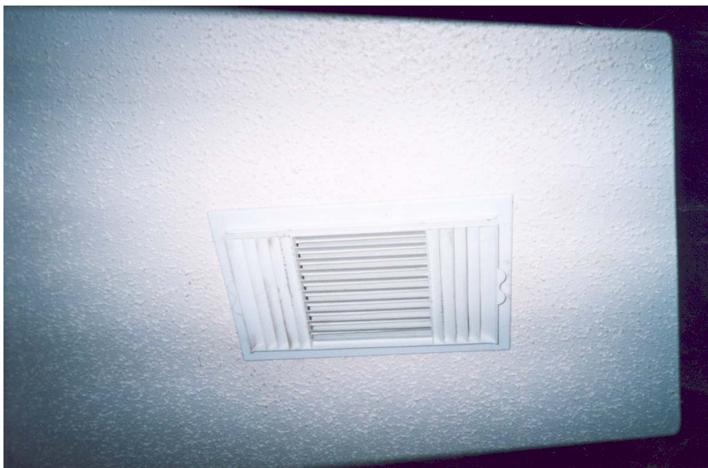
PHOTO 4: Additional view of minor buildup on an HVAC outlet vent.
