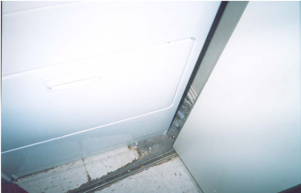
PHOTO 6: View of dirt buildup on the floor of the Laundry Room.
