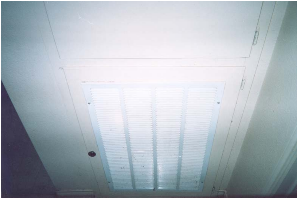
PHOTO 2: View of minor dust buildup on HVAC return air grill.
