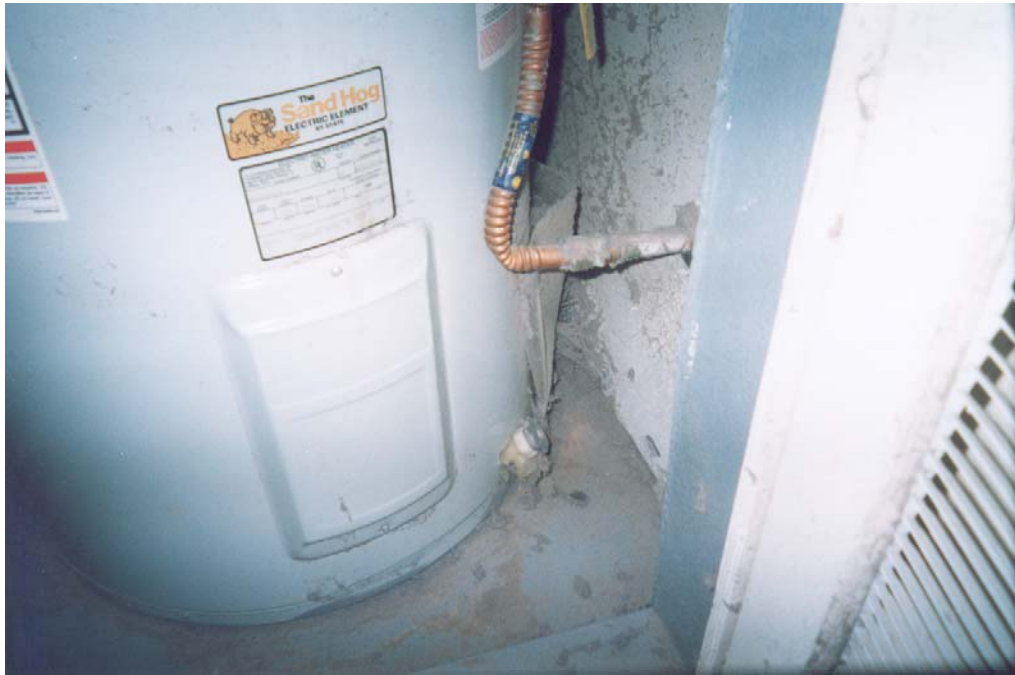
PHOTO 5: View of excessive dust buildup inside the water heater closet which is also the return air duct.
