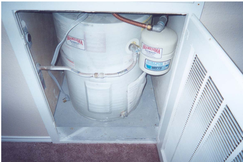
PHOTO 2: View of return air vent and water heater closet.
