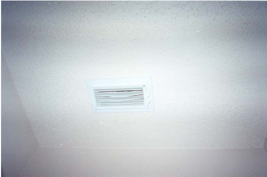
PHOTO 1: View of typical HVAC outlet.
