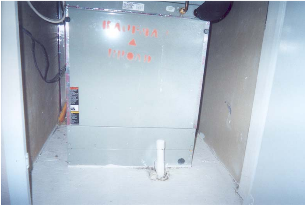
PHOTO 3: View of HVAC closet.
