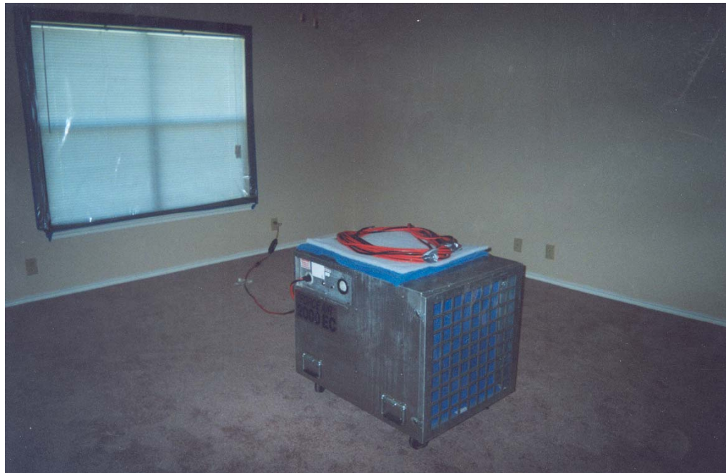
PHOTO 2: View of air scrubber in Living Room.
