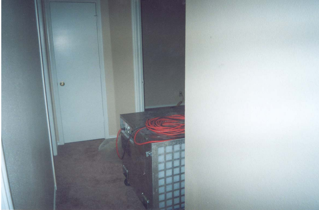
PHOTO 3: View of air scrubber in Hallway.
