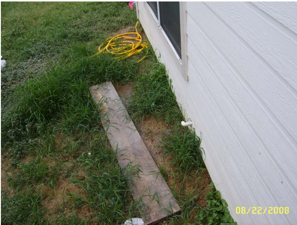
A/C condensate line - water pooling
