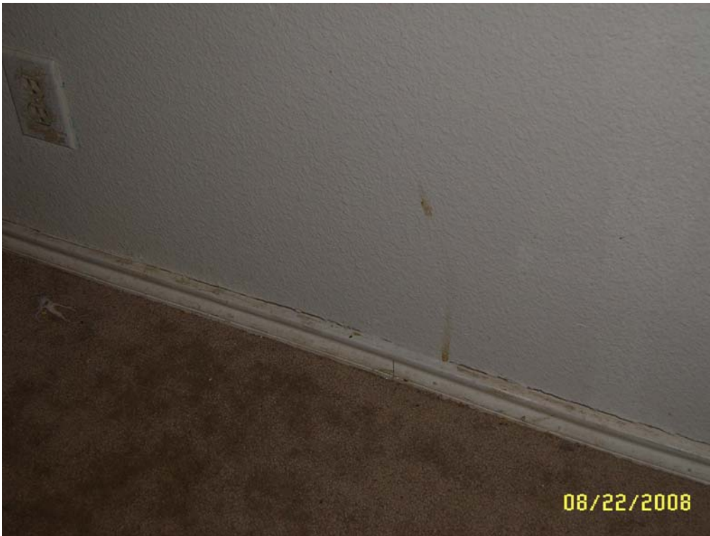
Living Room wall backing condensate line
