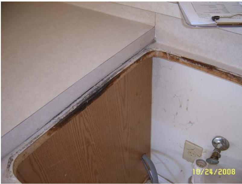
Kitchen countertop - discoloration
