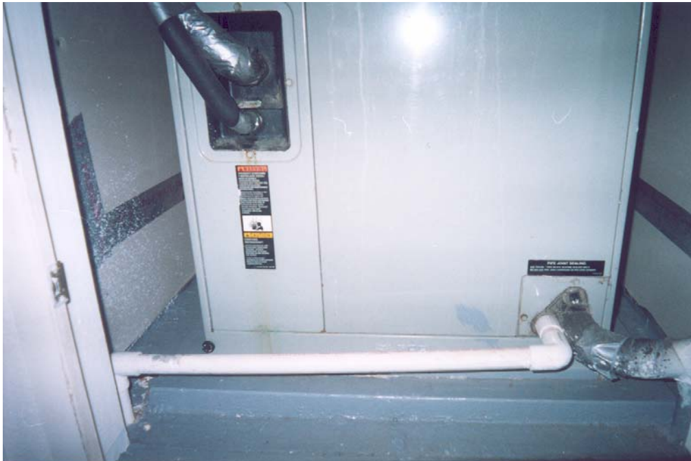
PHOTO 8: View of generally clean HVAC unit closet.
