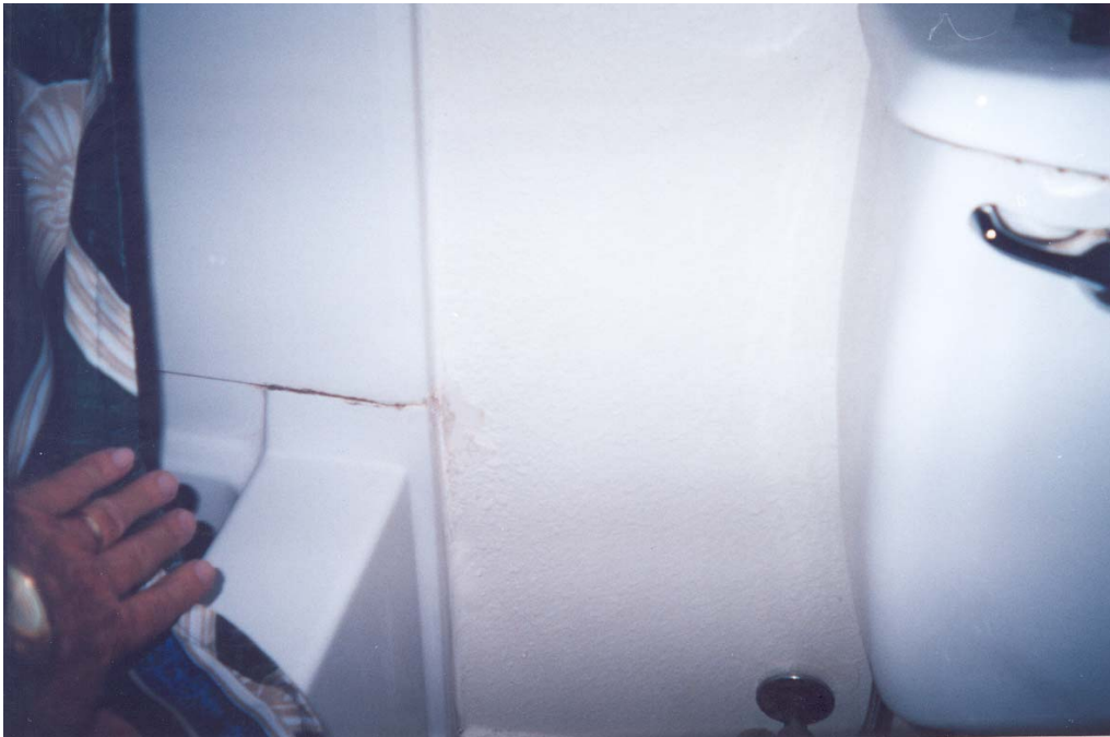
PHOTO 6: View of area where moisture is present in the sheetrock.
