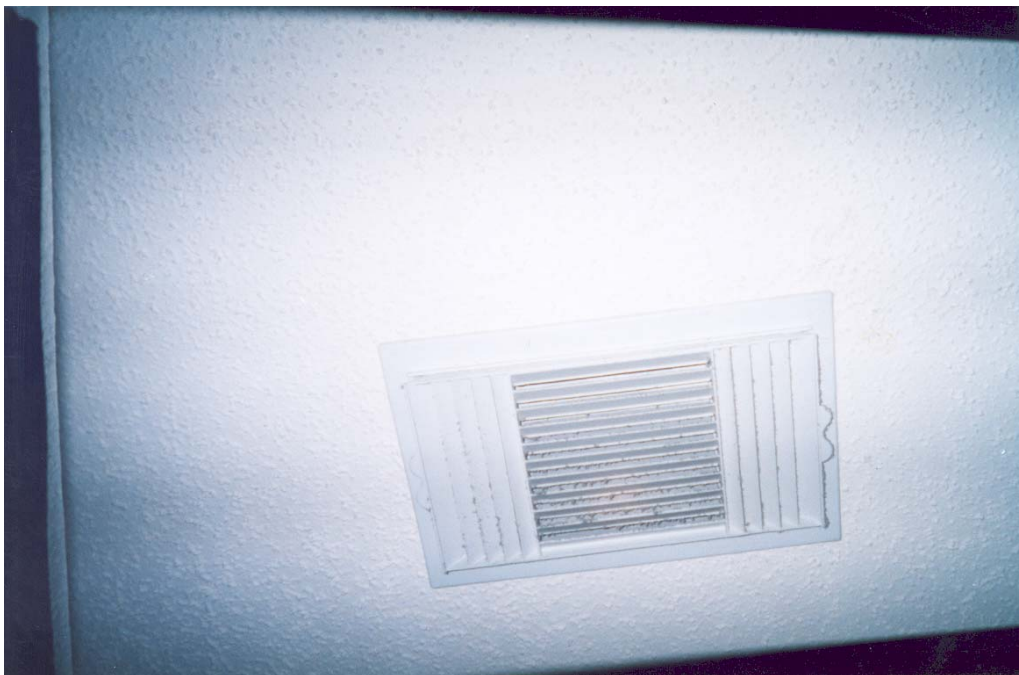
PHOTO 4: Additional view of buildup on an HVAC outlet vent.
