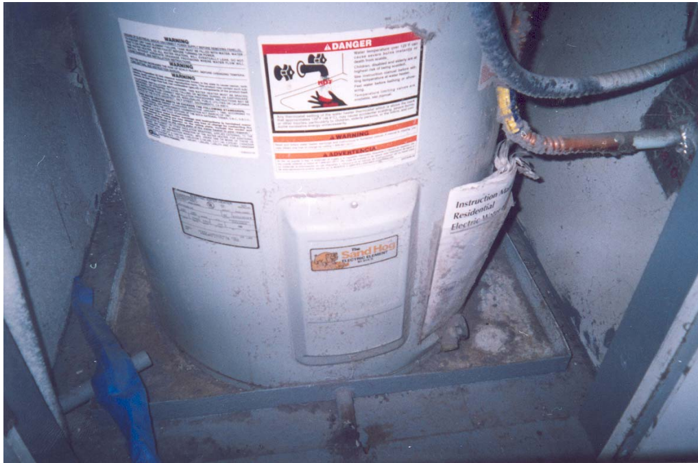
PHOTO 7: View of dusty return air closet with water heater.
