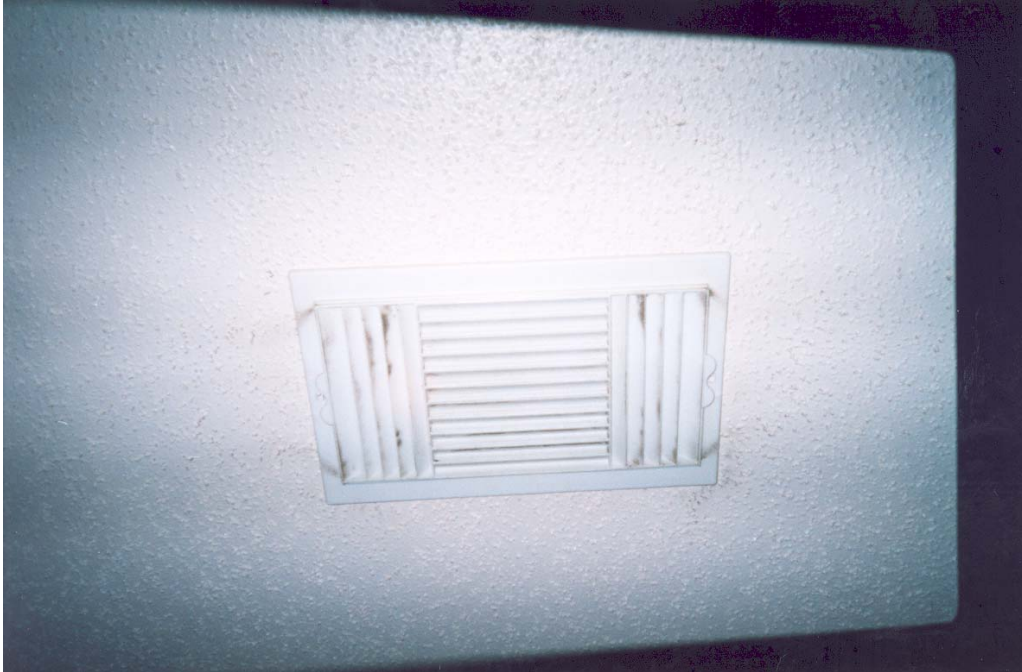
PHOTO 3: View of buildup on HVAC outlet.
