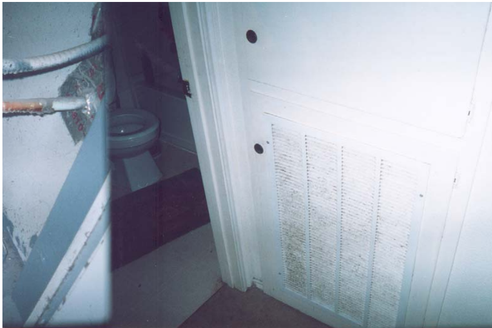
PHOTO 2: View of buildup on HVAC return vent.
