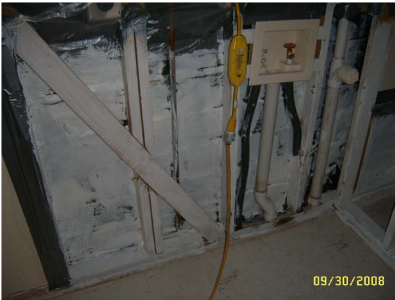
Utility wall at washer connection
