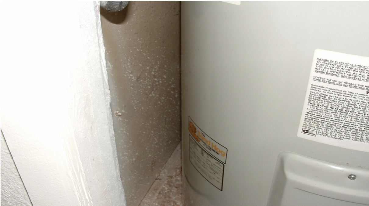
Photo 14: HVAC Closet- Return air plenum.
