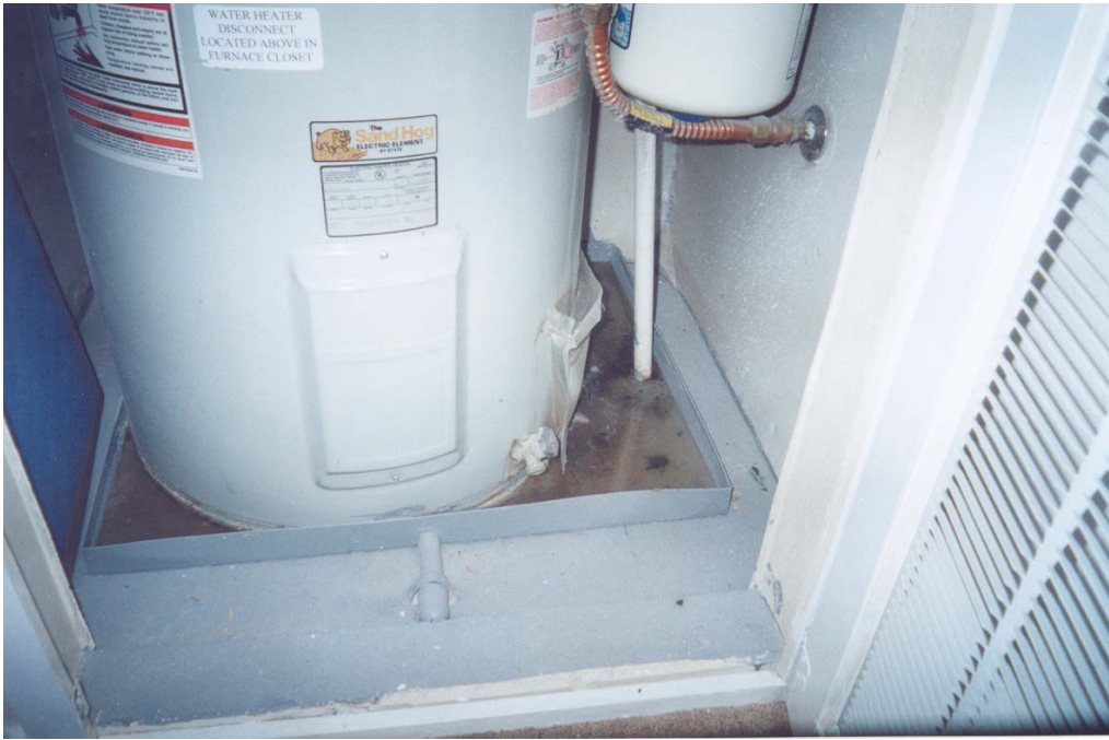
PHOTO 7: View of water in the condensate pan beneath the water heater.
