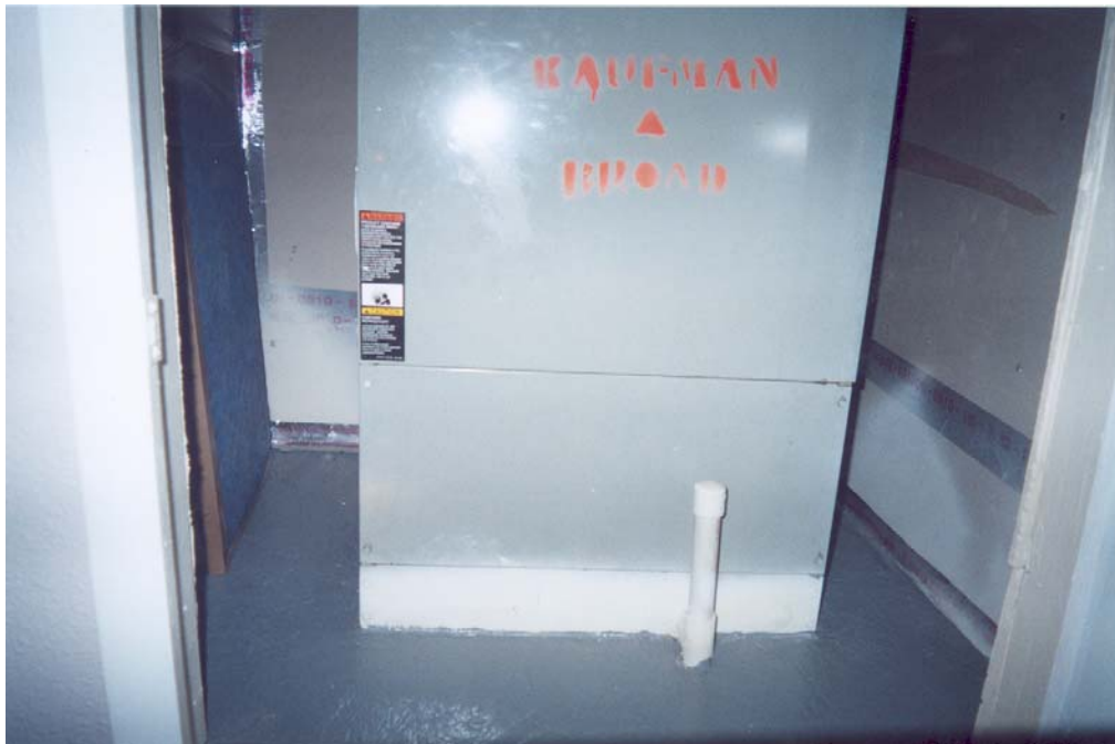
PHOTO 6: View of a clean HVAC closet.
