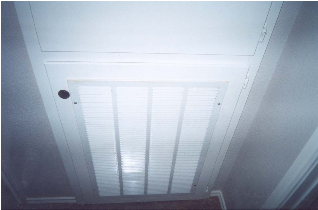
PHOTO 5: View of the clean HVAC return vent.
