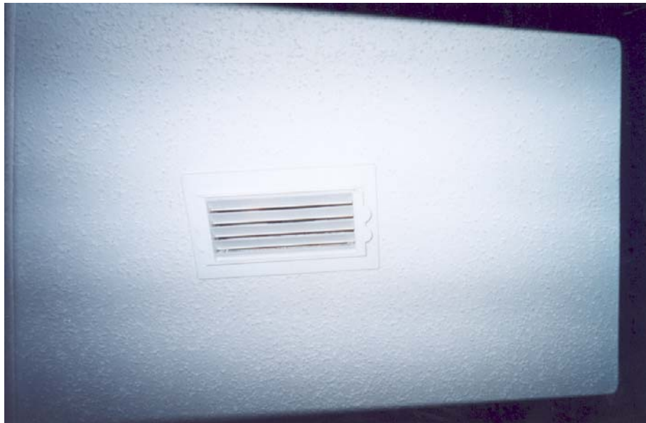
PHOTO 2: View of a clean HVAC outlet.
