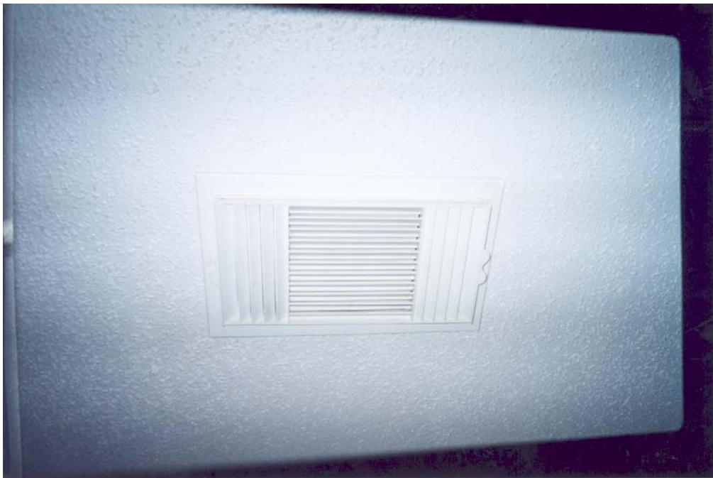
PHOTO 4: Another view of a clean HVAC outlet.
