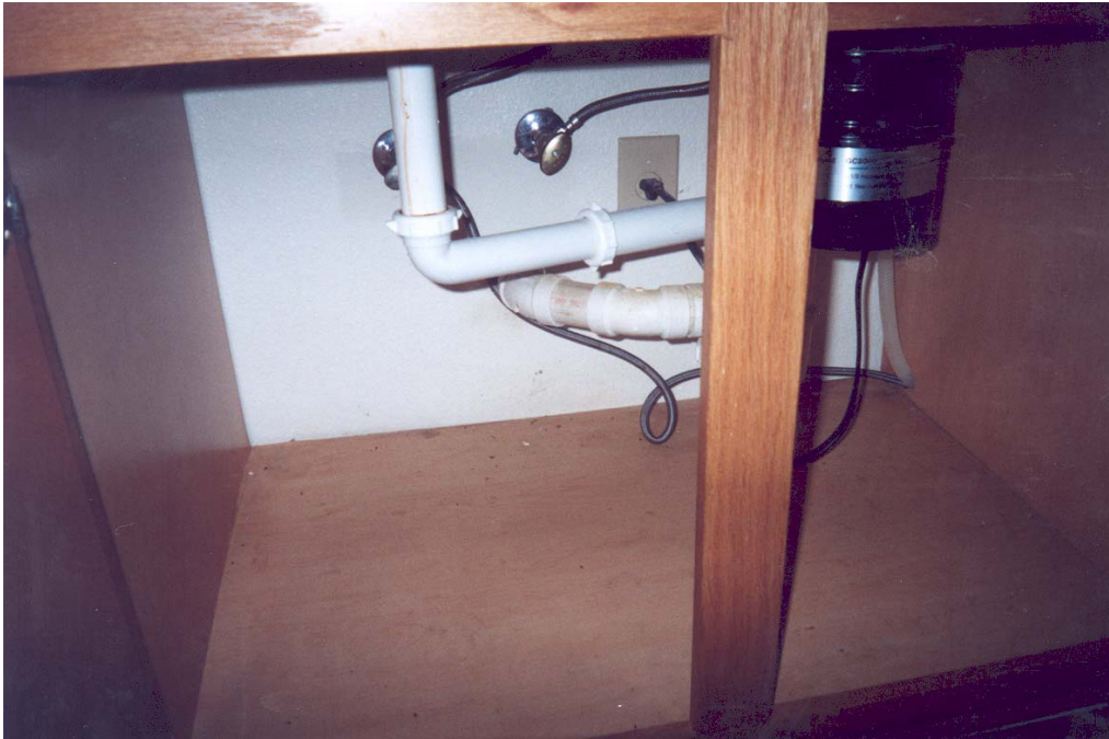
PHOTO 9: View of dry but dusty area under the sink.
