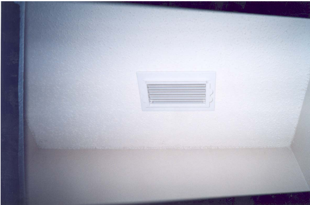
PHOTO 2: View of a clean HVAC outlet.
