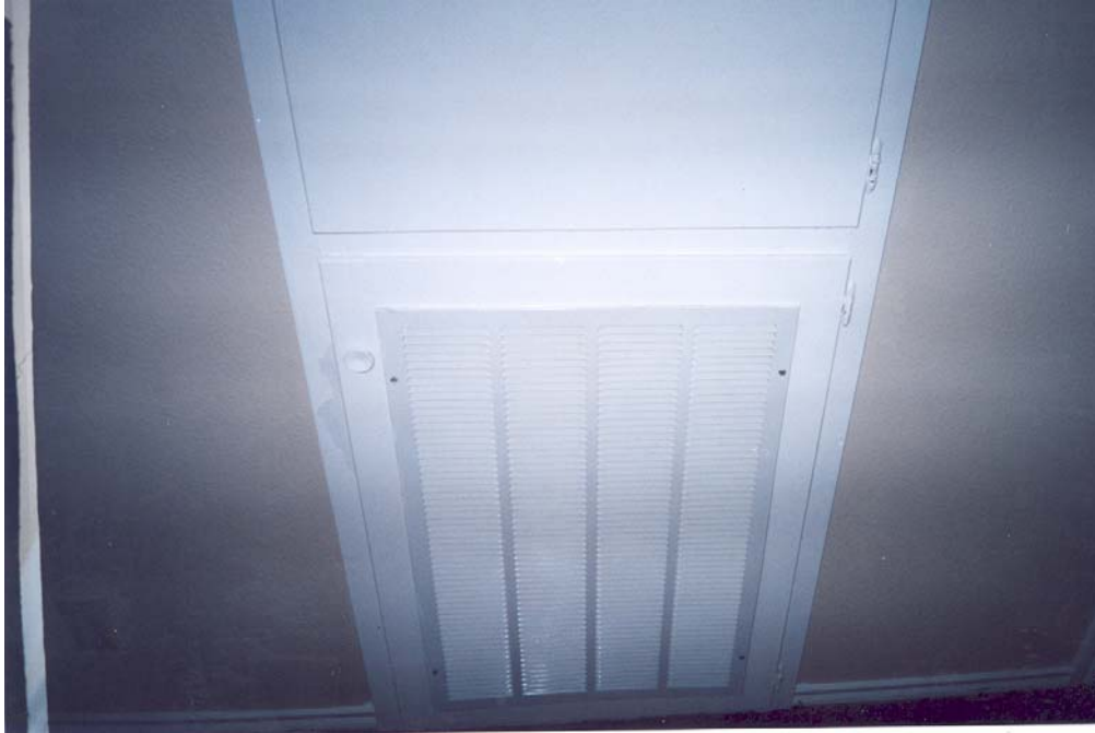
PHOTO 1: View of a clean HVAC return air vent.
