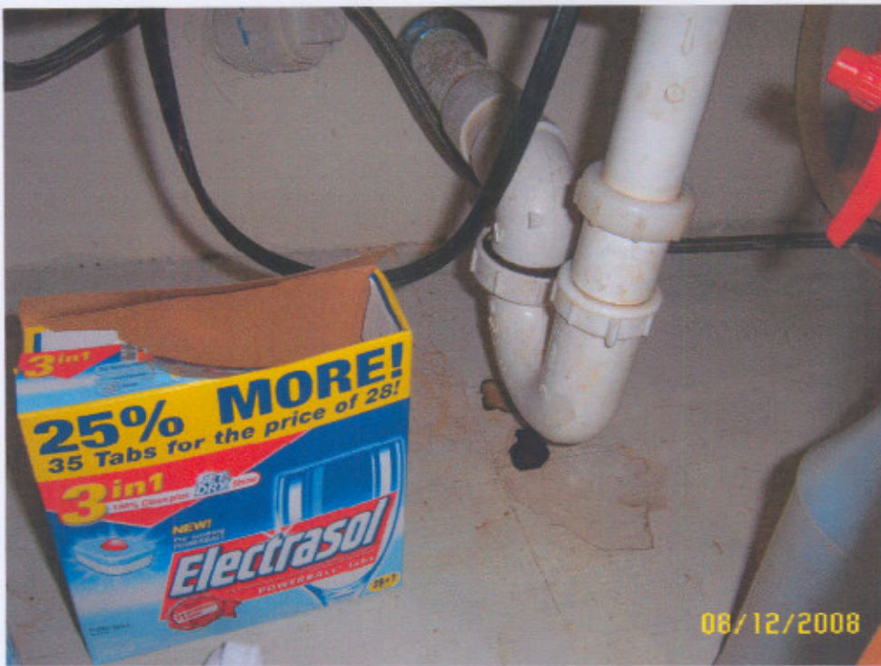
Kitchen - shelf below sink with water present on drain connection
