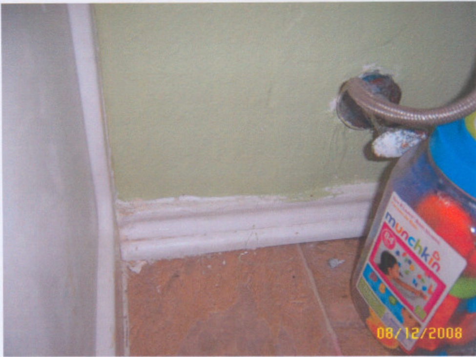
Hall Bath - sheetrock behind toilet
